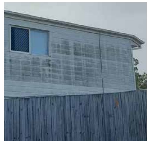
An example of Mould before treatment
